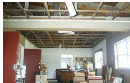
The Admin offices after Hurricane Ivan
